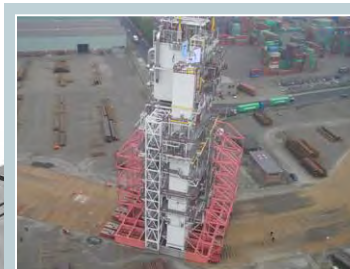
Fabricom Cold Box: 3 100 tons
