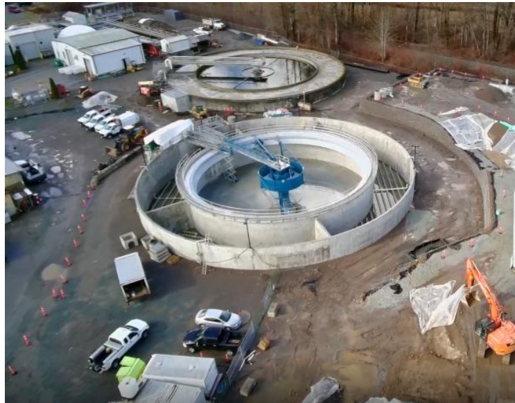
Figure 19: Clarifiers at Mamquam Wastewater Treatment Plant.
