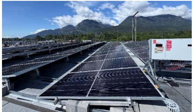
Figure 22: Rooftop Solar PV at Tantalus Firehall.
