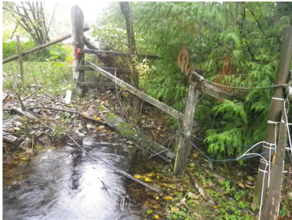
Photo 4: Looking north at the connection between west ditch and north ditch. October 23, 2014.
