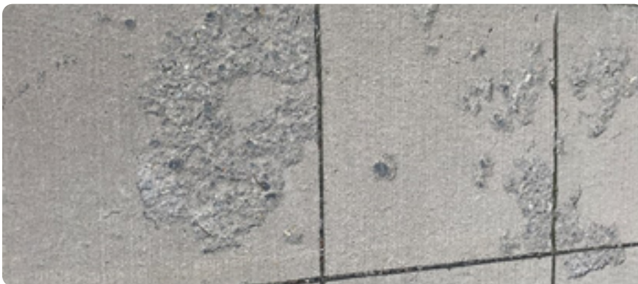
Fig 2.10.2) Shows salt damage to new concrete after the use of salt products over one winter season.
