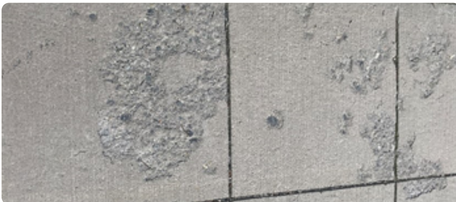
Fig 2.10.2) Shows salt damage to new concrete after the use of salt products over one winter season.
