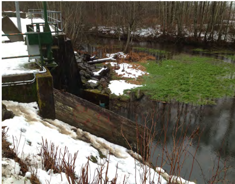
(Figure 6.2): Judd Slough Pump Station. A mechanical artifact in the wilderness.
