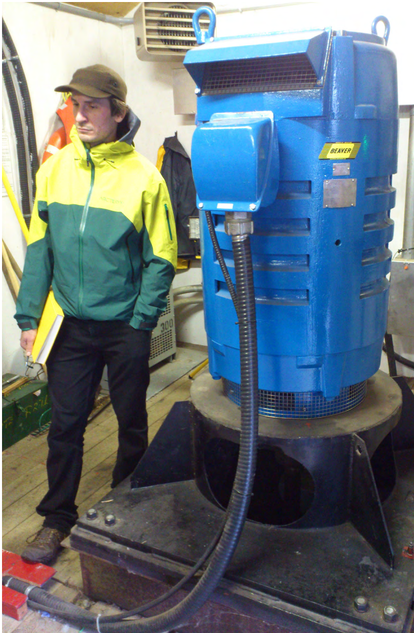
(Figure 5.13): One of two second-hand pump units in station 1 & 2 (in the shack).
