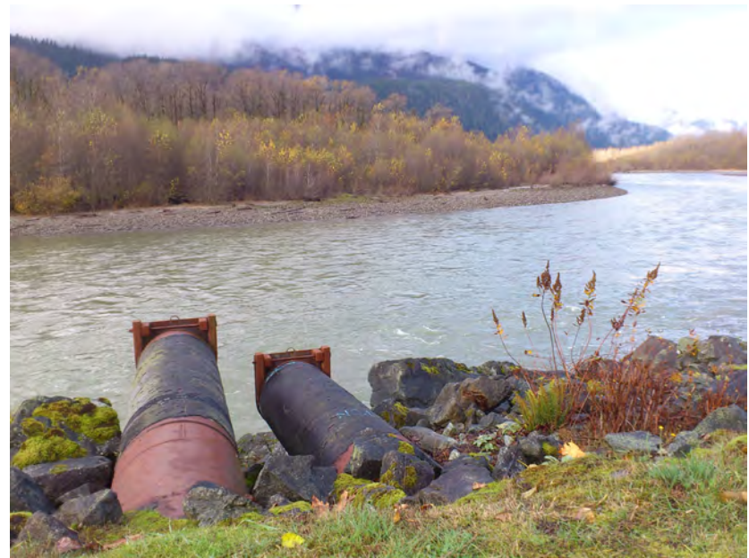
(Figure 5.14): Station 1 & 2 outlet pipes to Squamish River
