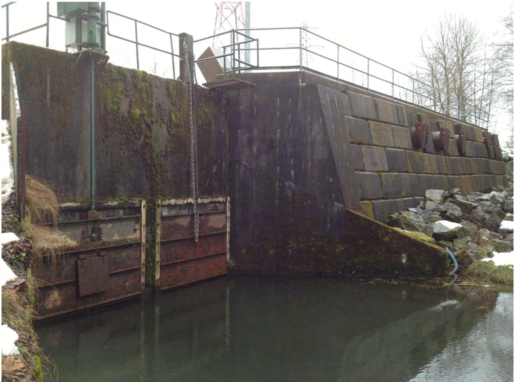
(Figure 6.3): The rugged, concrete wall at Judd Slough Pump Station speaks to the scale of engineering required to live in this powerful region.
