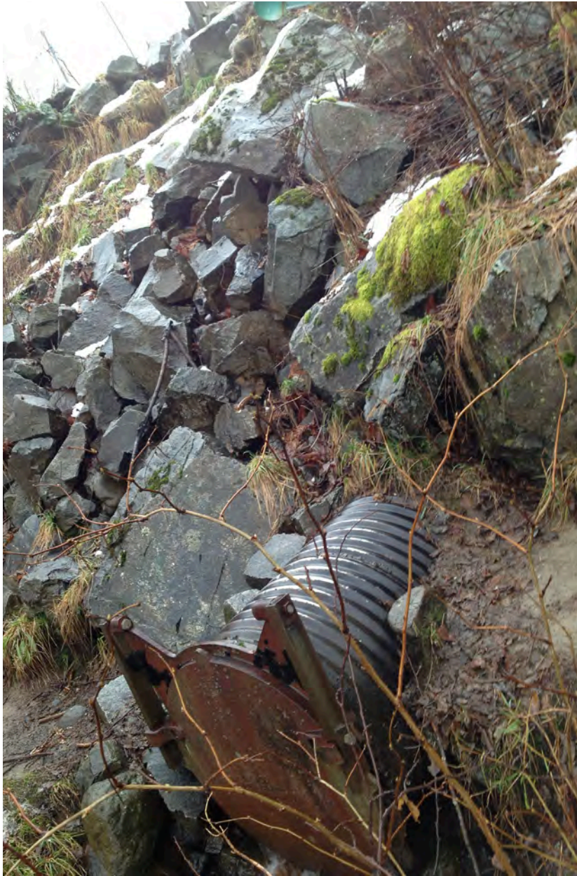
(Figure 6.4): Horse Creek Outlet protrudes from the dike at the Brackendale waterfront edge.
