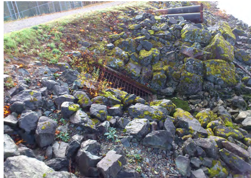
(Figure 5.16): The rusted gate in the foreground is the outlet for the “Big Bertha” VFD’s.
